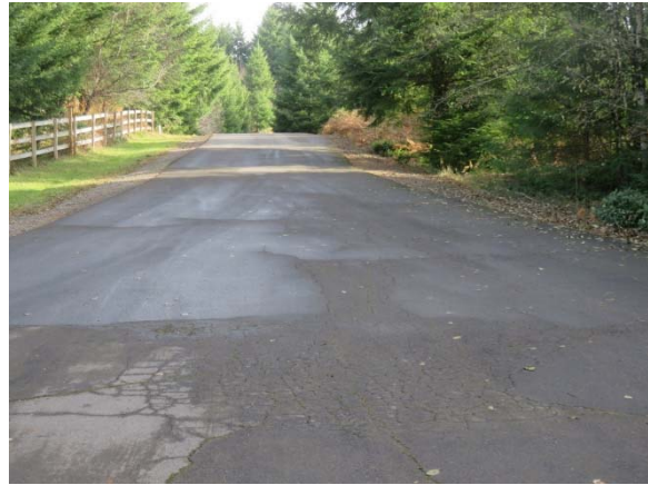
Typical Area of Asphalt Damage
