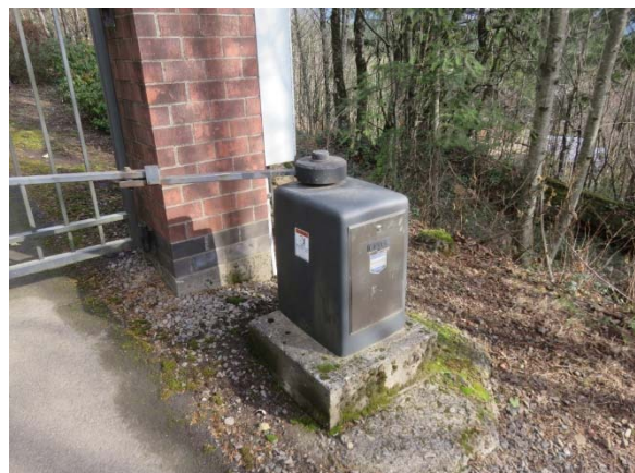
One of Two Gate Operators at Gate #3
