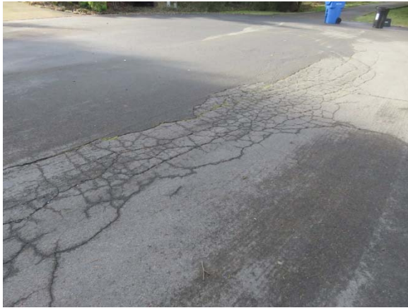
Typical Area of Asphalt Damage
