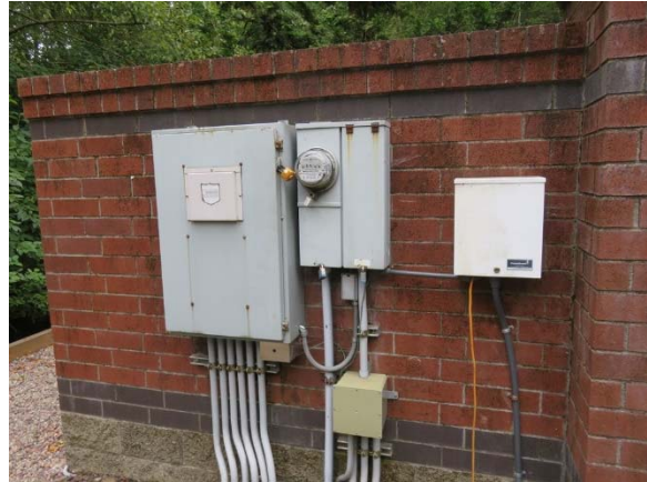
Electrical Breaker Panel and Meter at Gate #1
