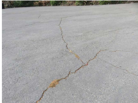
Typical Asphalt Cracking
