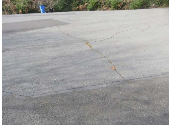
Typical Area of Asphalt Damage in Need of Repair
