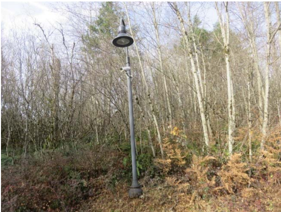
One of Six Pole Mounted Lights
